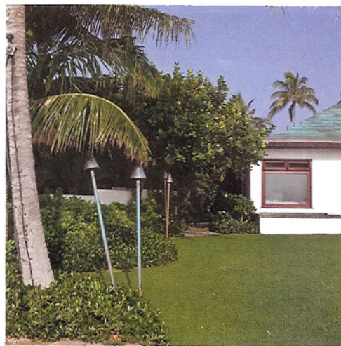
Left: Dewald installed low-voltage lighting fixtures throughout the property to promote energy savings.
